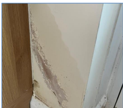
Picture 1: Rising damp to side of kitchen unit on external wall.
