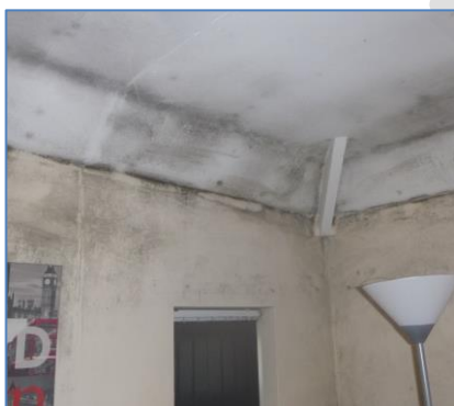
Picture 4: Black spot mould following condensation to walls and ceiling.
